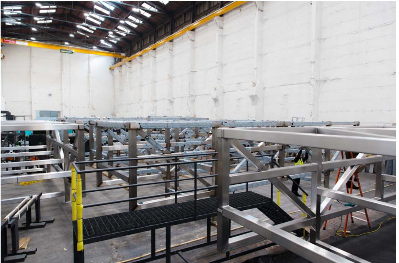
Stephen Cummins carrying out video inspections of weld penetration on stainless structural steel.
