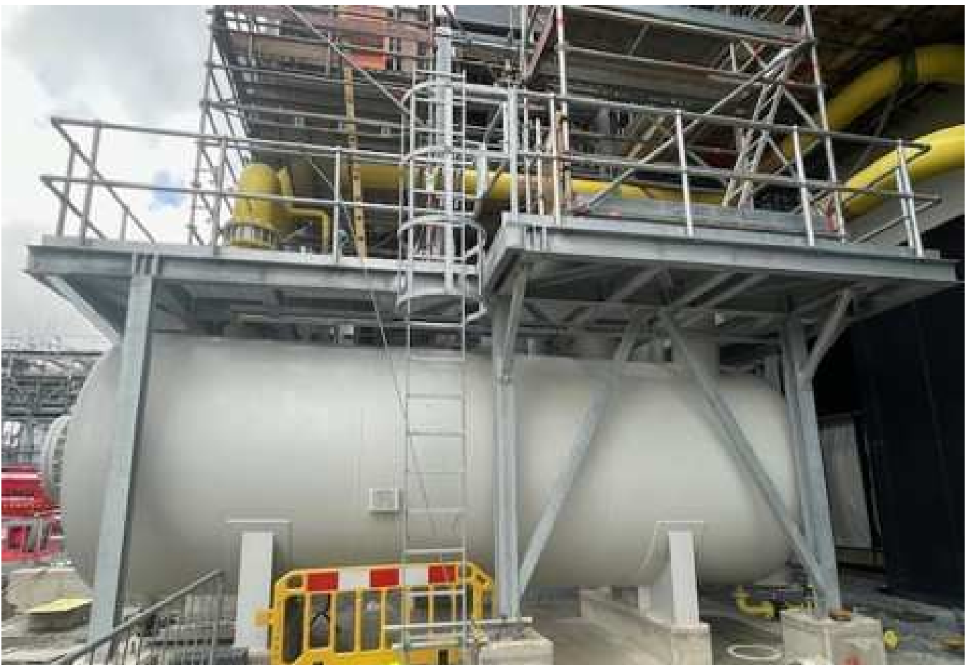
Astrazeneca Dublin. OMC installed stainless steel access platforms, Access stairs, Access ladders, lifting beams and galvanised access platforms.
