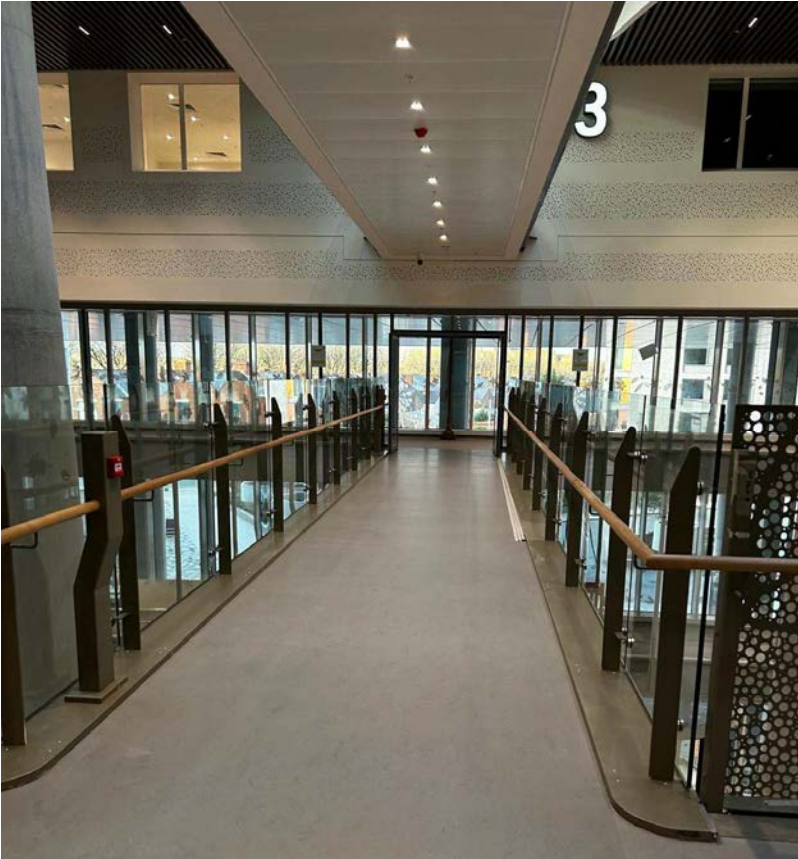
Various balustrade type's and flashings from around the hospital. Bridge balustrade, external glass balustrade and access pedestals.
