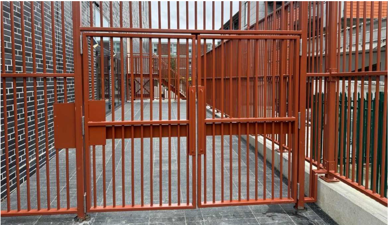
Galvanised and painted access gates, railings, and entrance screens to DCU Dublin.
