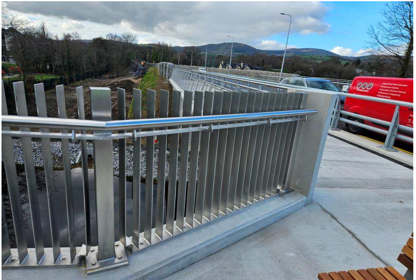
OMC supplied and installed Stainless Railings and seating to the viewing areas.
