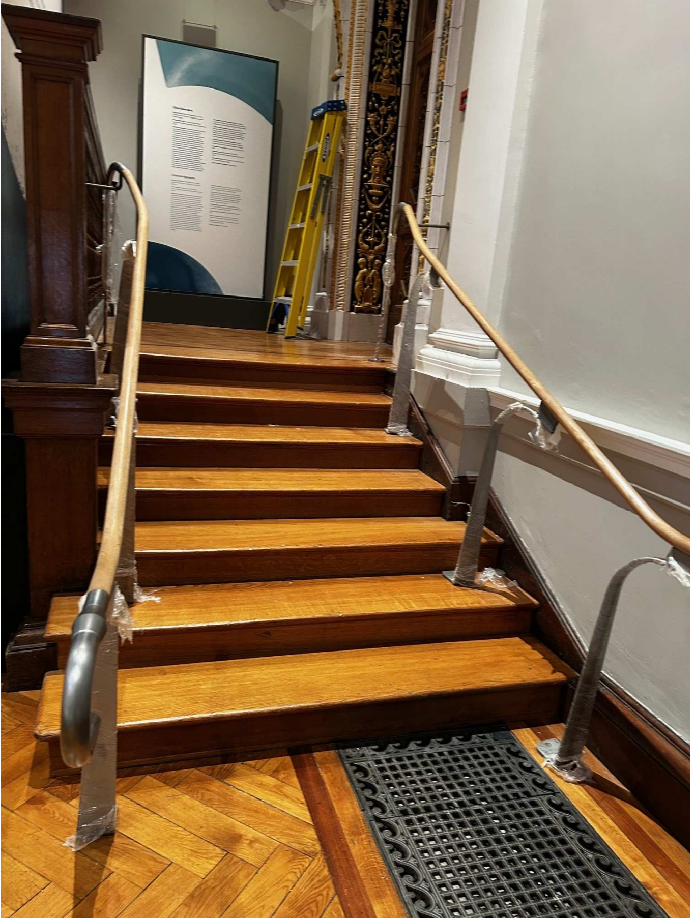
Polished and formed stainless steel uprights with timber handrails fitted recently in the National Gallery of Ireland, Dublin.
