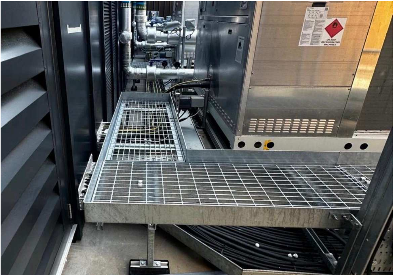
Galvanised roof access walkways, steps and railings. Plant access with no roof fixings.
