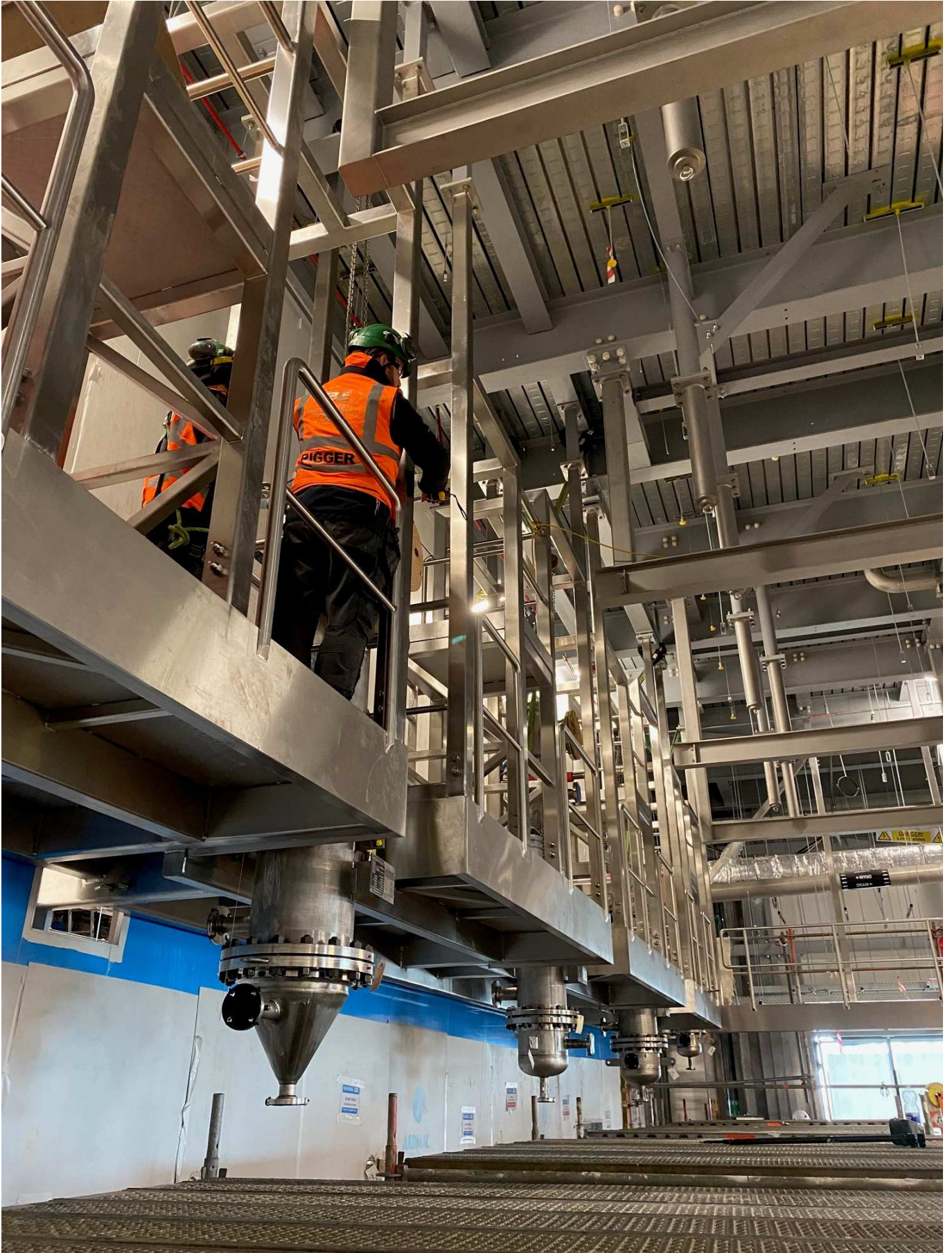
Astrazeneca Dublin. OMC installed stainless steel access platforms, Access stairs, Access ladders, lifting beams and galvanised access platforms.
