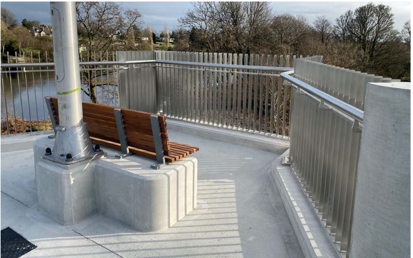
OMC supplied and installed Stainless Railings and seating to the viewing areas.
