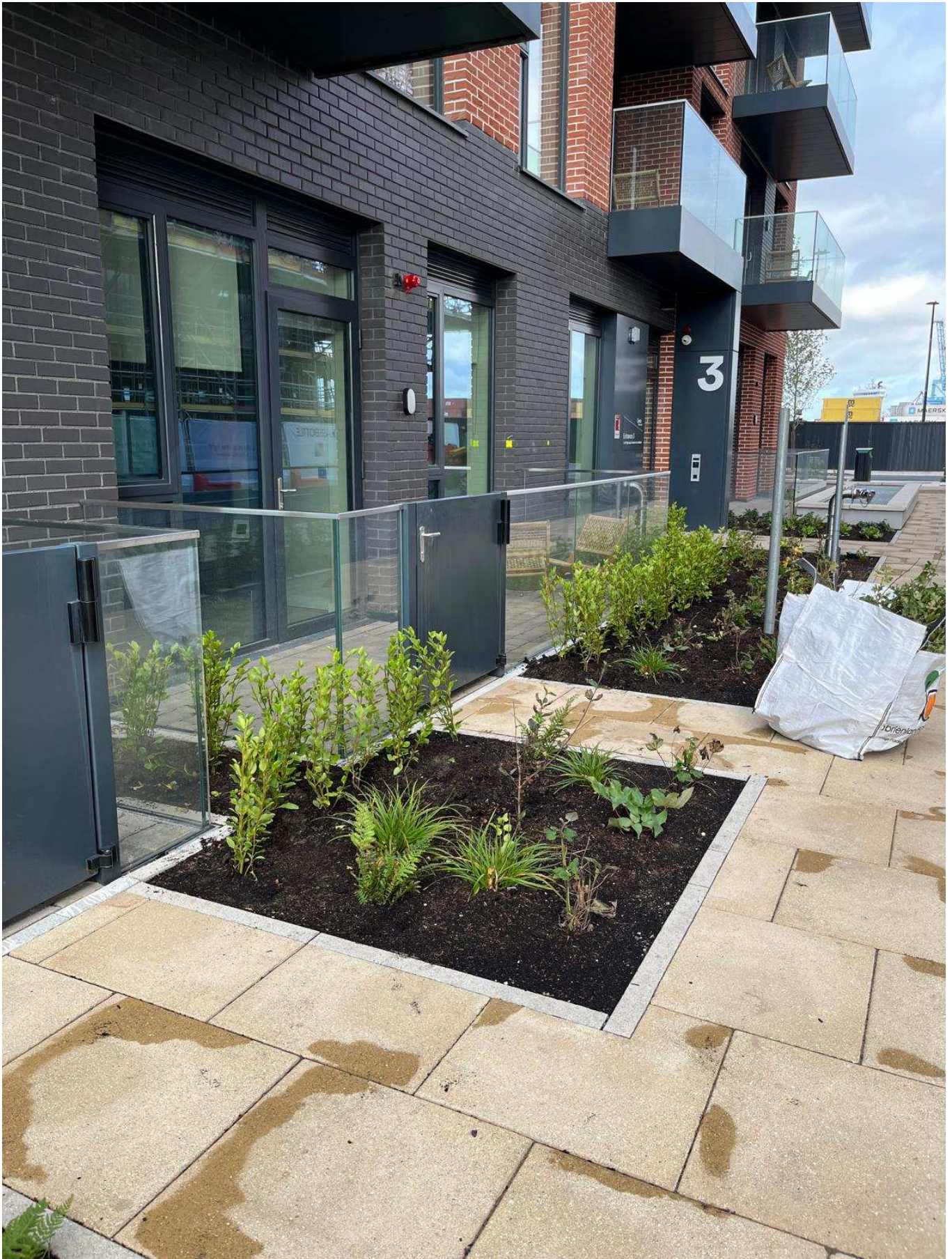
Glass balustrading with integrated PPC access gates fitted with lock's and closers.
